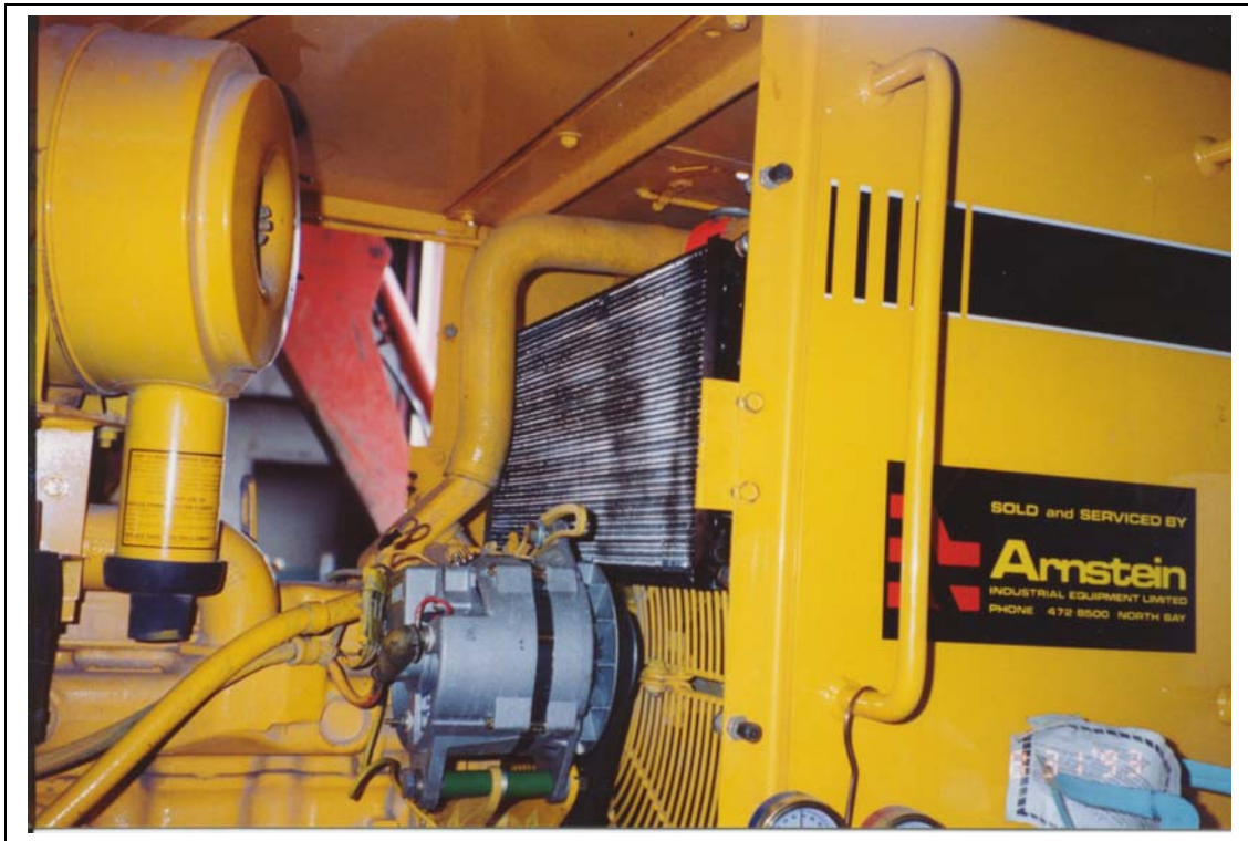
Right side of condenser
